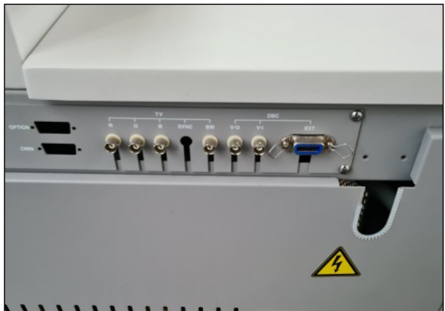
Video I/O (HV tank)
